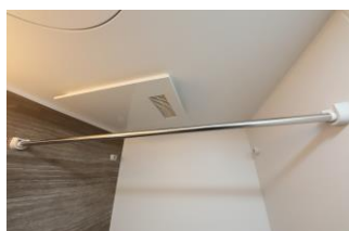
Dryer in the bathroom
